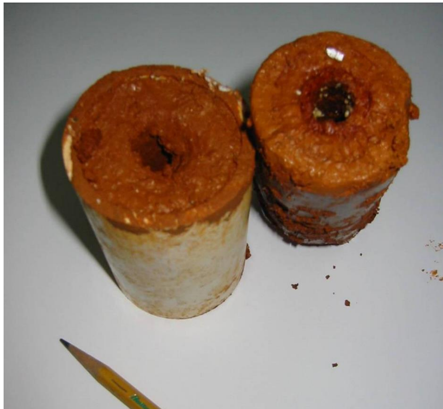
Figure 6. Dewatering pipe encrusted with iron and iron bacteria after approximately four months.
