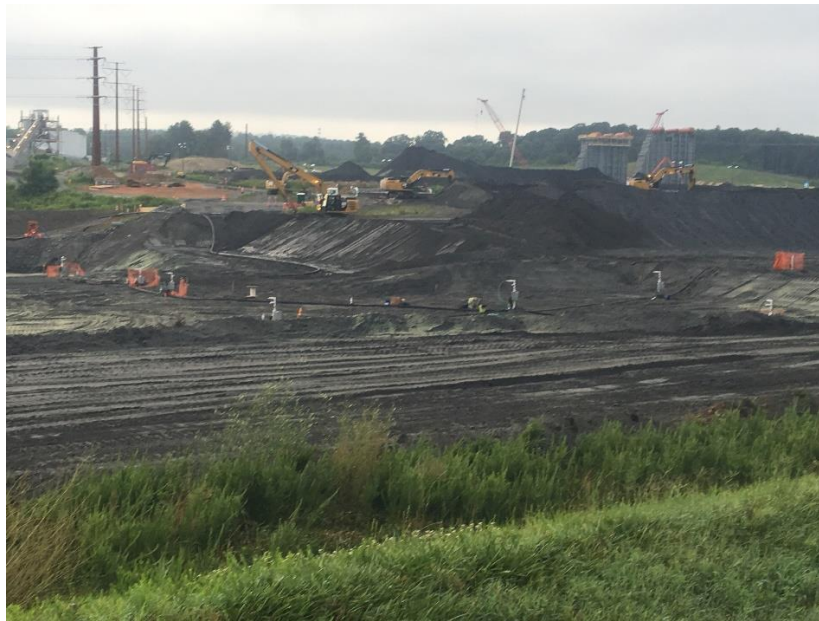
Figure 2. Widely spaced deep wells in a CCR impoundment.
