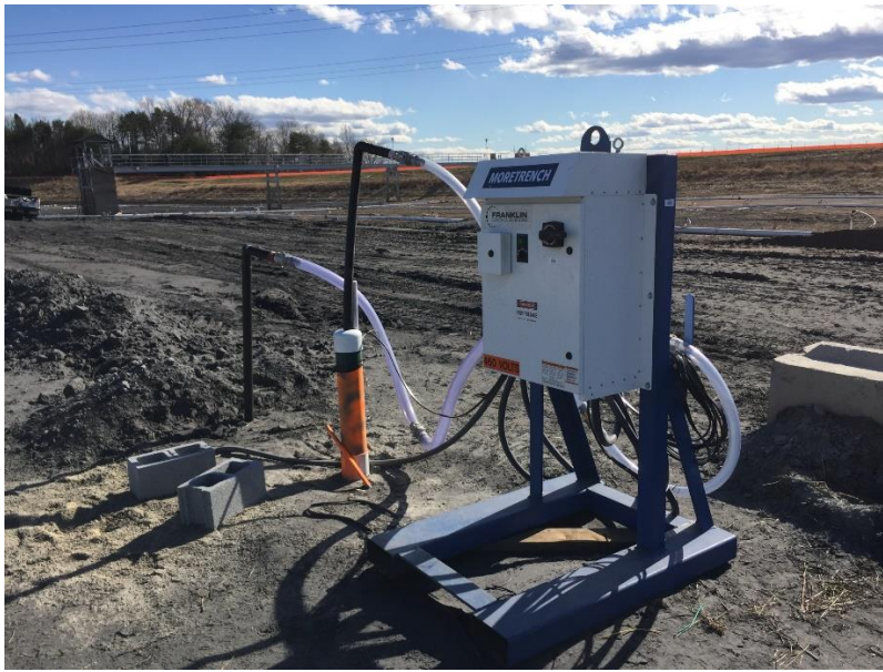
Figure 7. Deep well on CCR with a VFD control panel.
