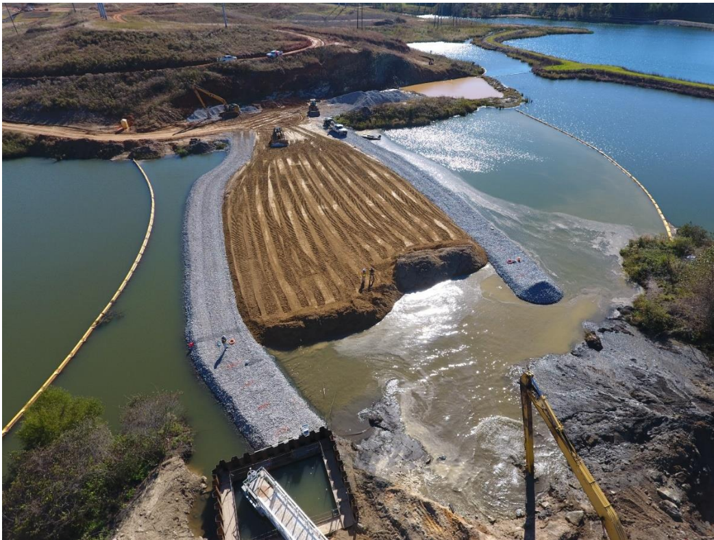
Figure 5. A significant thickness of new fill on a subaqueous soft pond bottom
