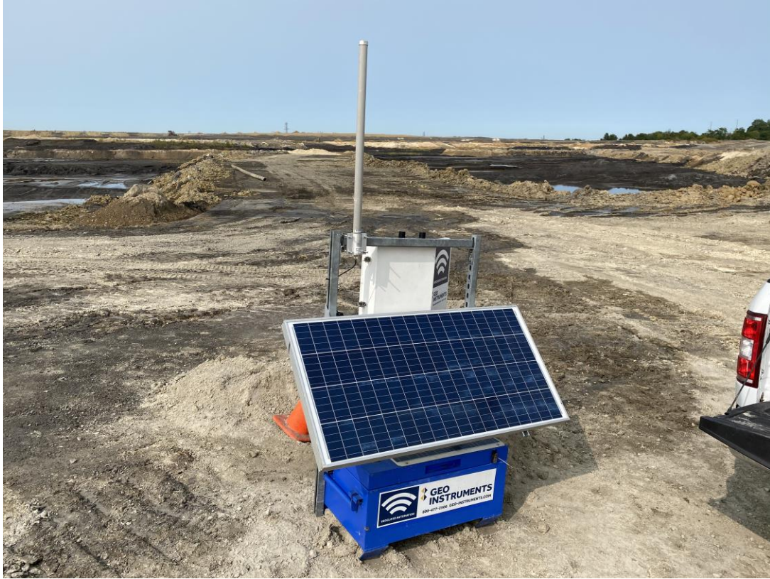
Figure 6. In order to safely put 18+ metric ton (40,000+ lb) drill rigs out on the gypsum, vibrating wire piezometers were installed and tied into a “spike sensor”
