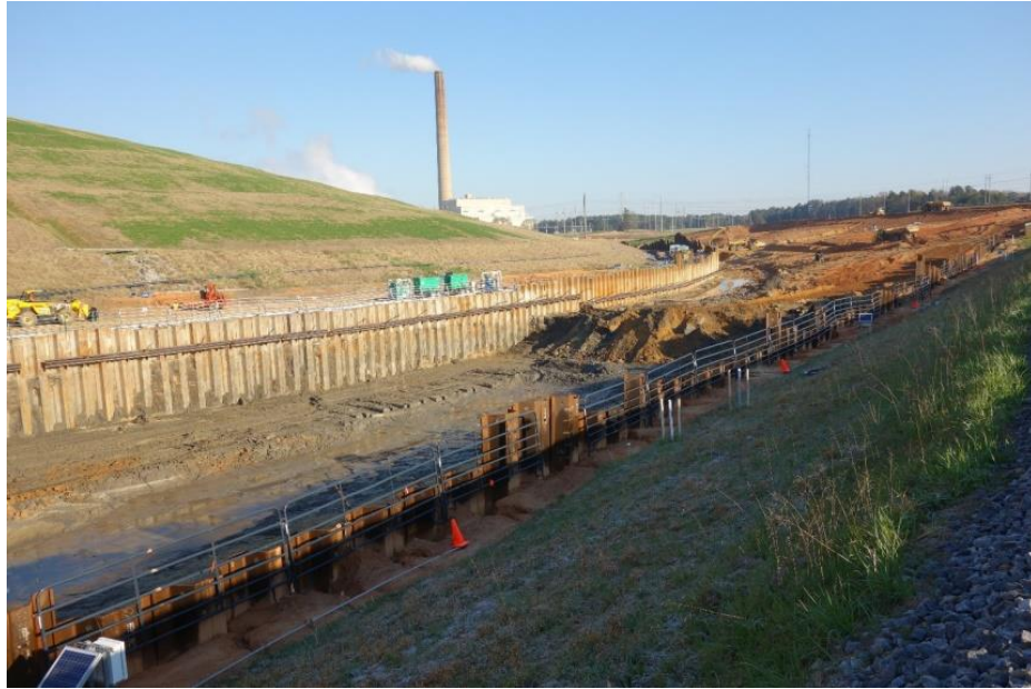
Figure 2. Support of excavation installation involving steel sheet pile driving and drilled tieback anchor installation.
