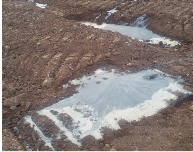
Figure 1. Sand boils associated with liquefaction in an ash pond
