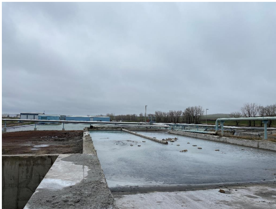
Figure 3. Sedimentation Basin System
