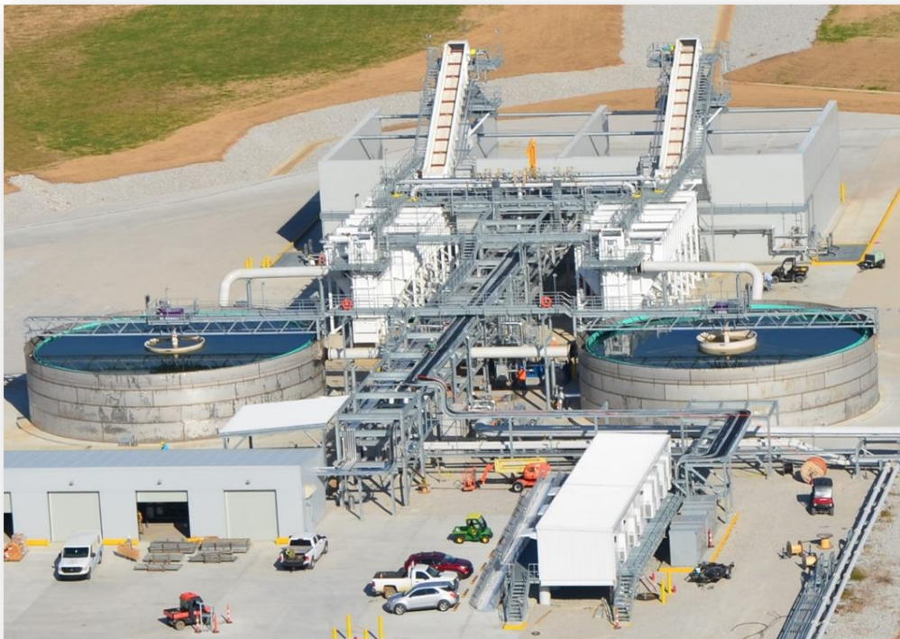
Figure 4. Remote Submerged Flight Conveyor Bottom Ash Dewatering System
